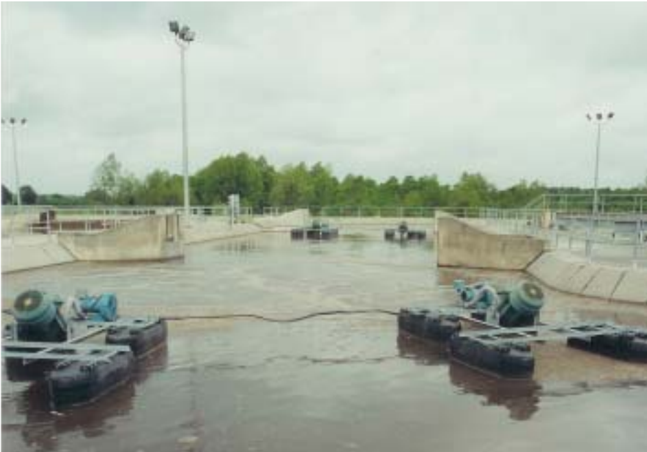
Triton aerators at the Franklin Wastewater Treatment Plant help to produce an effluent BOD of 2 to 3 mg/l.
