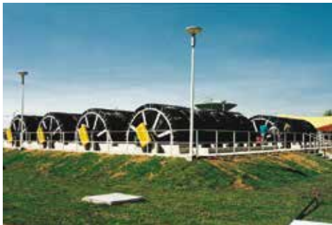
Large RBCs for biological treatment.
