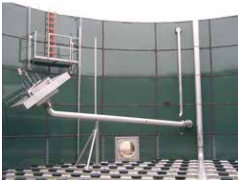
The decanter and access manway of a fruit juice wastewater treatment SBR Plant.
