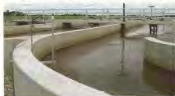
A closer view of the DO probe location on the west side of the oxidation ditch and the bridge mounted process aerator/mixer units.
