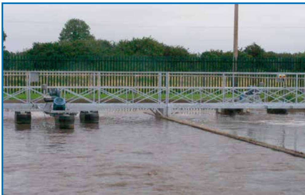
3.7kW Tritons® on a tri-pontoon float in position and fastened to the access gantry. The Triton® can be bridge or side-wall mounted.
