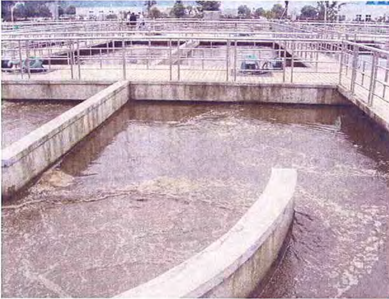
The Aire-O 2 Triton® aerators are bridge-mounted at Lin An for easy access.
