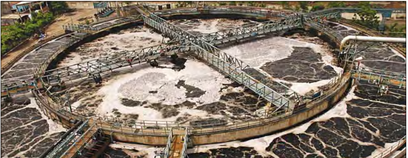
Triton aerator/mixers at Green CETP, Vatva, Ahmedabad, using 12 x 60HP Triton aerator/mixers, is one of the biggest installations in India
