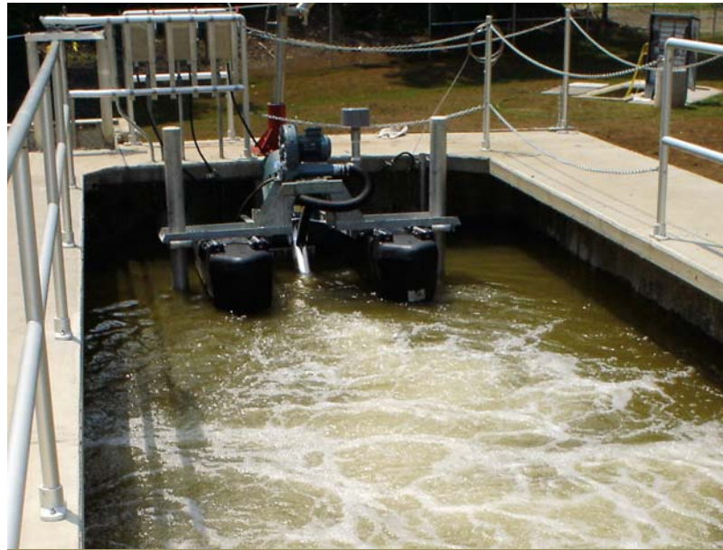
The Triton dual-function aerator/mixer provides process flexibility to nitrify and denitrify as well as facilitate biological phosphorus removal by changing controls to allow for anoxic mixing steps during the cycles.
