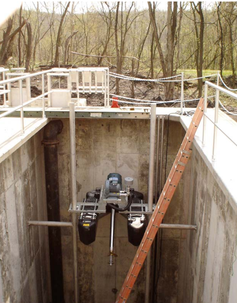
This pre-start up photo shows how the unit is able to ride vertically up and down on stainless steel slide-pole assemblies as water levels in the tank change.
