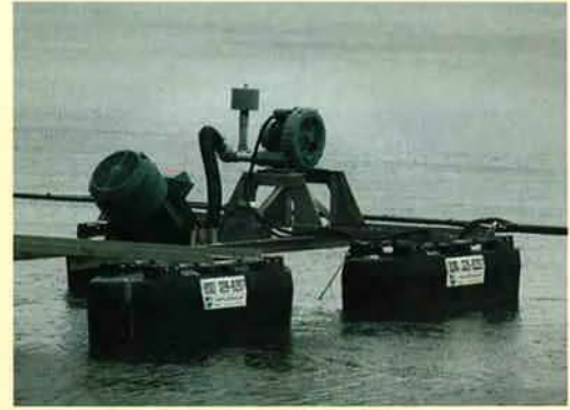
Aerators driven by energy-efficient motors, which are activated by oxygen sensors, help reduce energy use by nearly 60 percent at Astoria's wastewater treatment plant.
