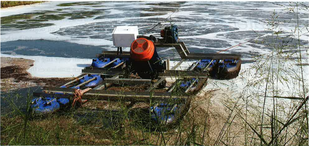
A 45kw Aire-O 2 Triton Aerator that was installed at Sappi - Stanger Mill
