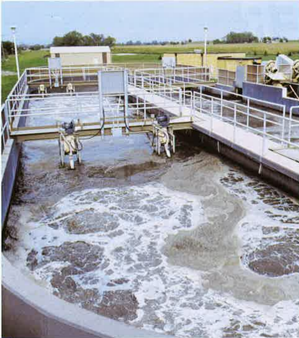
An Aire-O 2 Triton aerator/mixer shown in a bridge mount at an oxidation oval site in Europe
