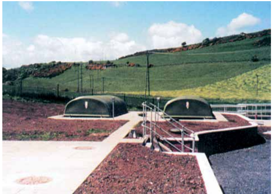
The newly installed DC17 RBC system at Auchtertool, UK.
