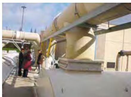
Air Extraction System for GRP Cover.
