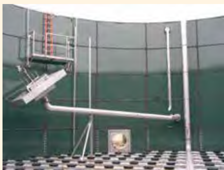
The decanter & access manway of an SBR at a fruit juice factory
