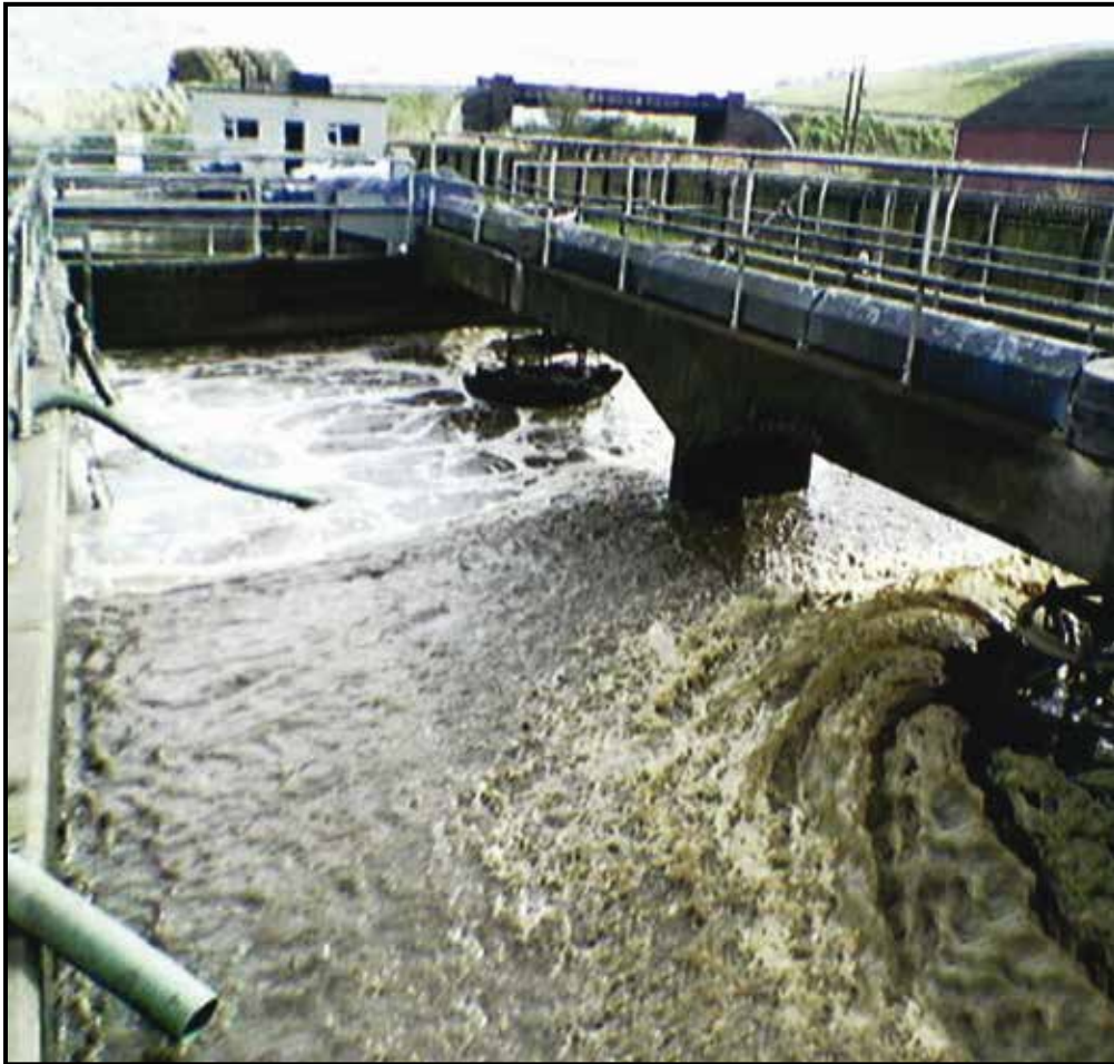
EXISTING AERATION SYSTEM NOT FULLY WORKING - ONLY ONE SURFACE AERATOR OPERATING
