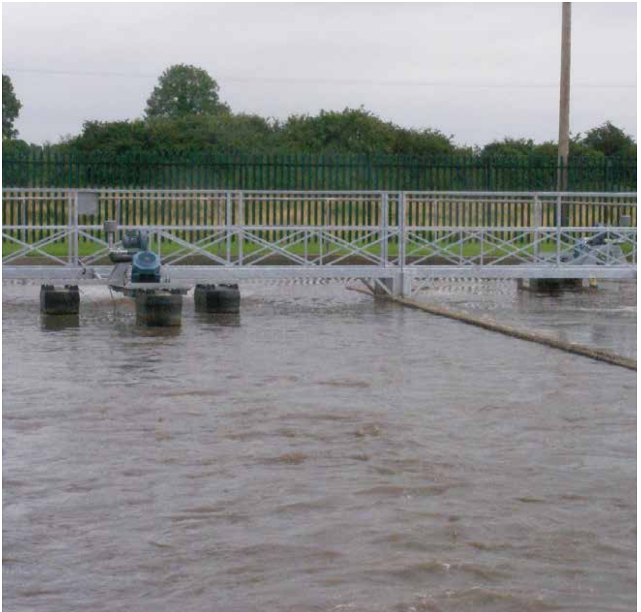
3.7kW Tritons® on a tri-pontoon float in position and fastened to the access gantry. The Triton® can be bridge or side-wall mounted.
